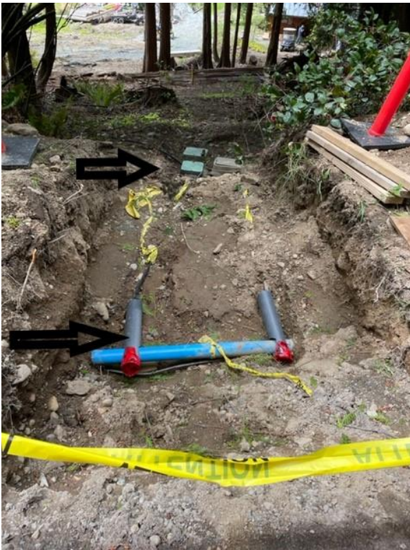
Bottom arrow is new installation to main water line and top arrow connects 3/4" hose to resident curb stop. Buried with sand and warning tape and valves covered with PVC pipes to protect valves.
