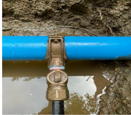
New Saddle Clamp and Valve connection with 3/4" hose running to a new curb stop.
