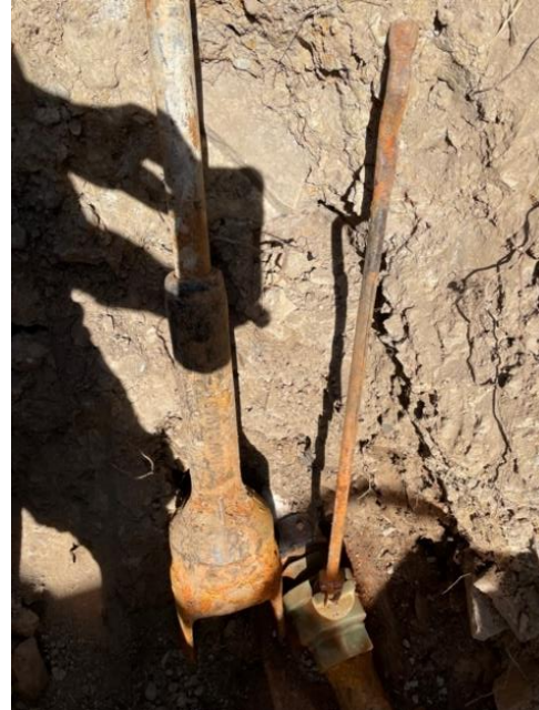
Metal shroud over Gate Valve. Metal extension fit inside tube and corroded.
