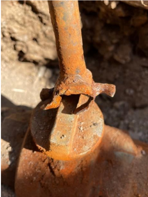
Extension metal bar that key was opening Disimilar metals corroded connection
